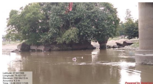
Figure 33: Debris of old Lodhipur bridge
